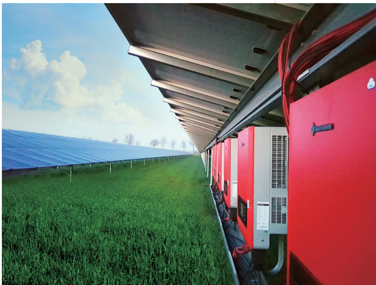
12MW Rotterdam | Holland
