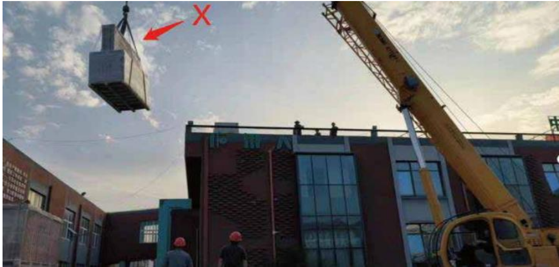
(Figure 10 Incorrect Diagram Illustrating Transportation of Stacked Boxes Using Crane)
